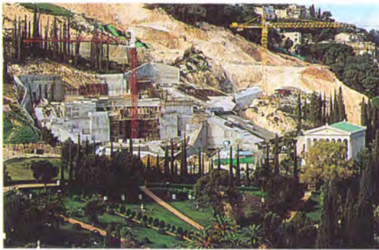
The almost completed structure of the Centre for the Study of the Texts is defined by its semi-circular entrance portico.
