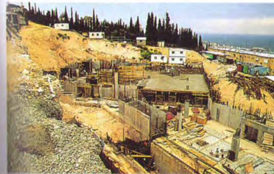
By March 1996 the structure of the International Teaching Centre had reached its second level.
