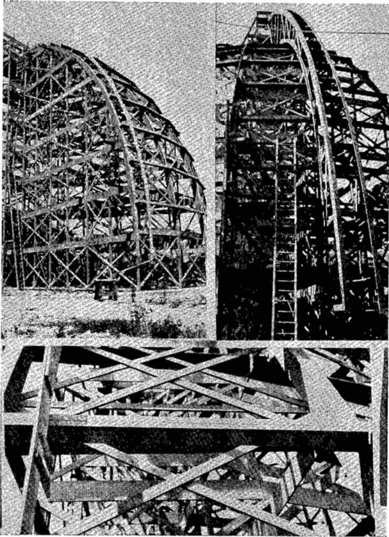
Figures 3, 4, and 5.—A scaffold supports timbers constituting a replica of the steel of a dome section.
