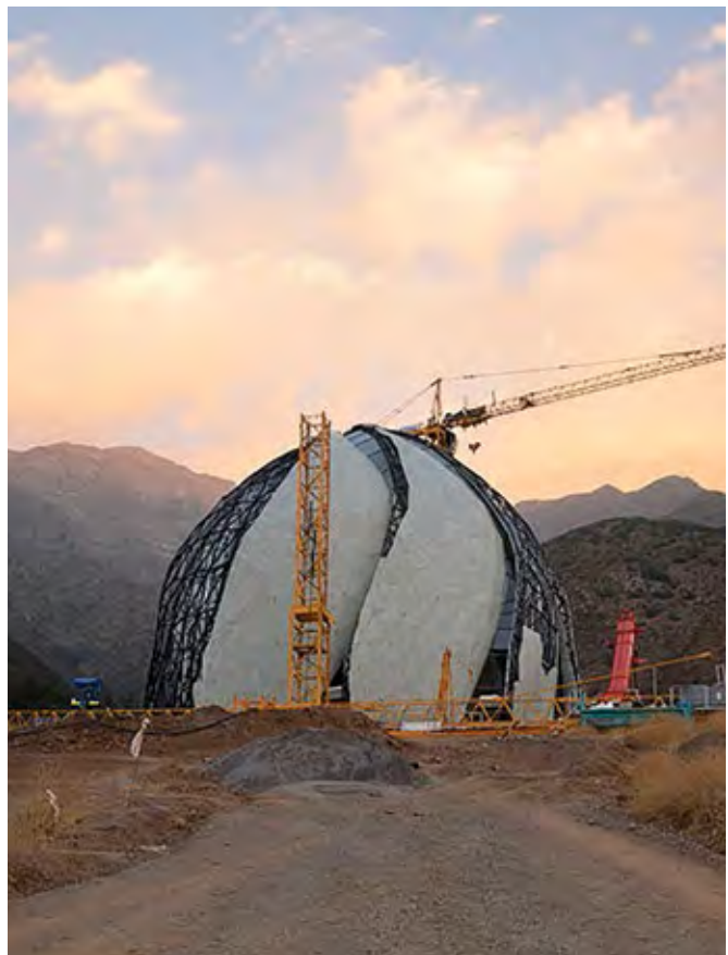
Construction advances on the Continental House of Worship for South America, in Santiago, Chile.
