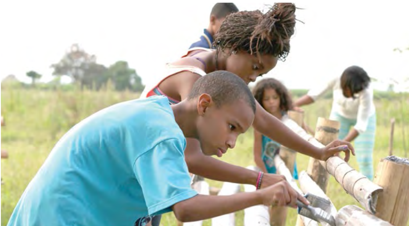
Youth contribute to the construction of benches near the land of the House of Worship in Norte Del Cauca, Colombia.
