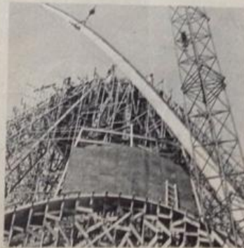
The present reinforced interior rib is being lifted into place to support the dome. The ribs are 1 1/2 inches wide for their full length but taper from a depth of eight inches near their lower intersections with one another to 2 1/2 inches at bottom and top.
