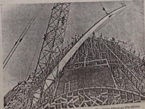
One of the fair-faced precast concrete internal ribs is lifted into place as the dome begins to take shape.
