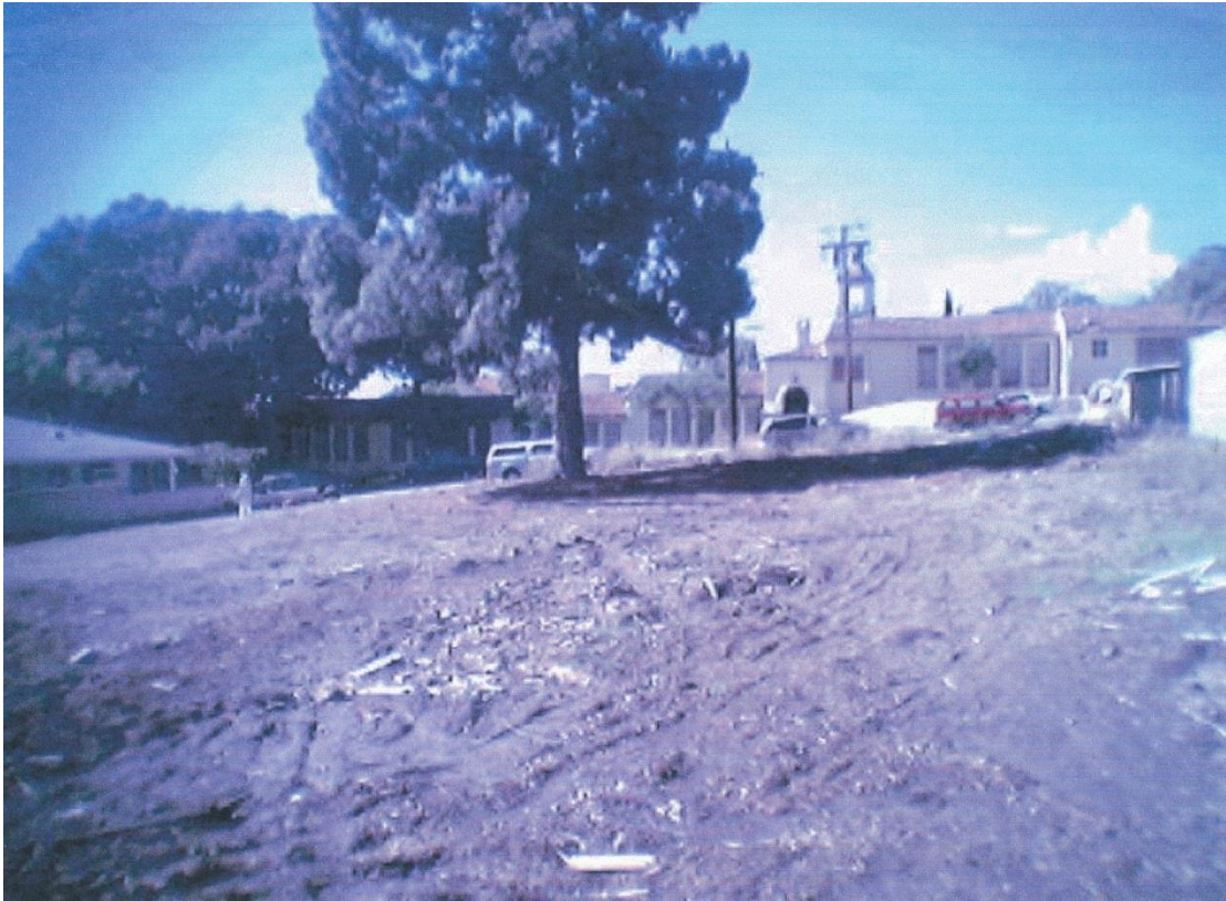
Sunny Slope property at 415 N. 6 th St. prepared for construction of new buildings, looking towards Santa Paula High School from the eastern side of the lot. This property was the site of the first Bahá'í residents and meetings in Santa Paula, and was called a "Mecca of Unity" from 1914-1944 when owners C.E. and Alma Elizabeth Carpenter lived there. In 1944 they moved to Berkeley to be nearer to their children.
